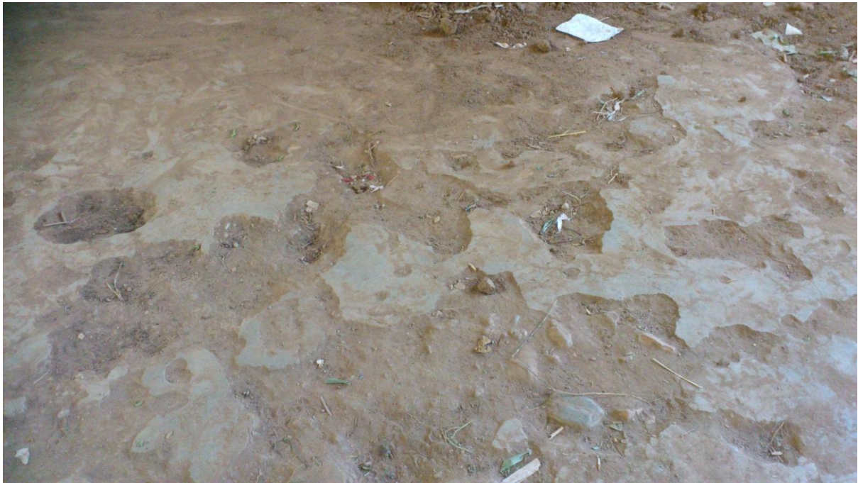
Plate 14: Poor state of classrooms
