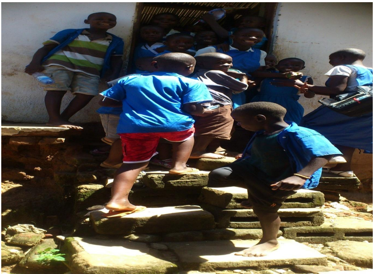
Plate 7: Sight of very Unsafe Entrance Areas
