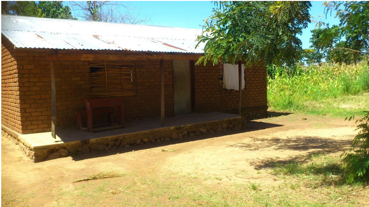
Plat10: Poor State of Teachers' Houses
