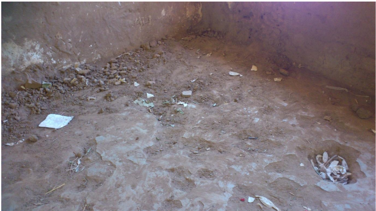
Plate 15: Poor state of classrooms
