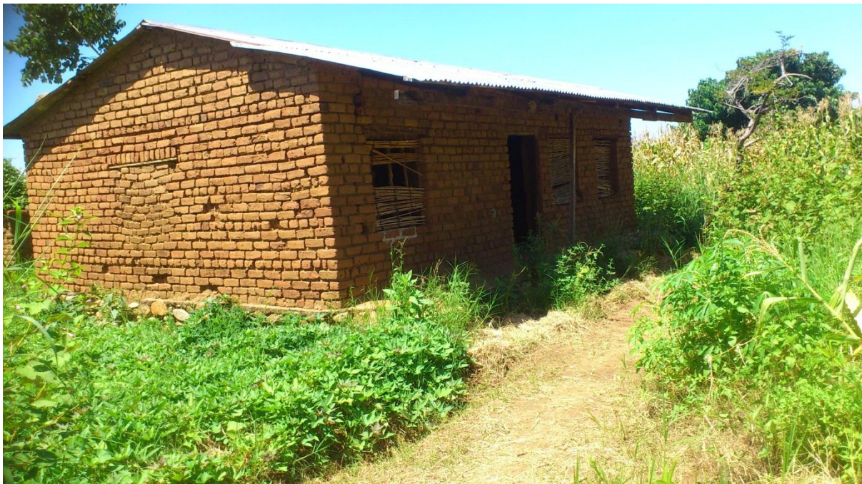
Plate 11: Poor State of Teachers' Houses
