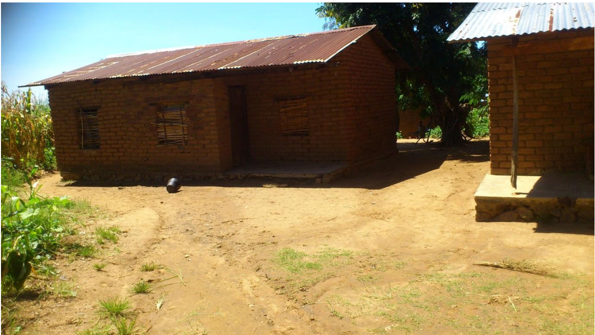
Plate 9: Poor State of Teachers' Houses
